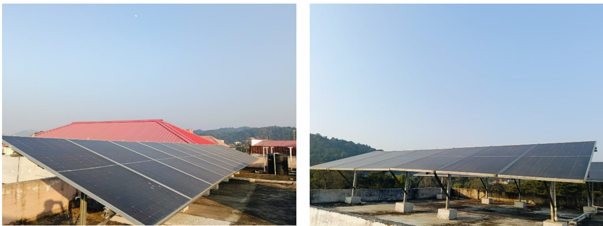
Figure 1: Rooftop hybrid Solar Photovoltaic (SPV) power plant.
